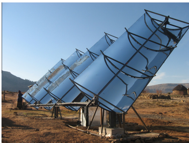
Fig. 1. Solar ORC prototype installed by STG in Lesotho.
