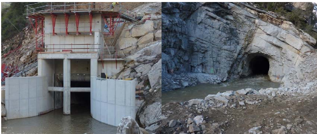
Figure 118: Actual inlet structure has been build according to the result of the design (left). The exit of the tunnel where the outlet still need to be constructed (right)
