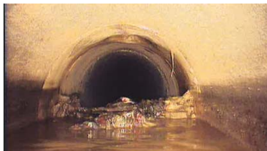
Figure 74: The endoscopy has revealed the presence of several obstructions
