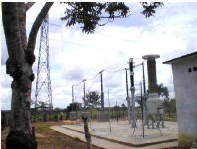
fig. 5 : The MAKOLA one-phase 50 kVA system. On the back, the 220 kV overhead line. On the front the LV house for the 230 V distribution to the population.
