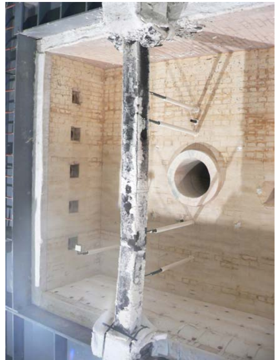
Fig. 6 Column 4B after the test
