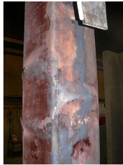
Fig. 4 Local buckling during test 4A
