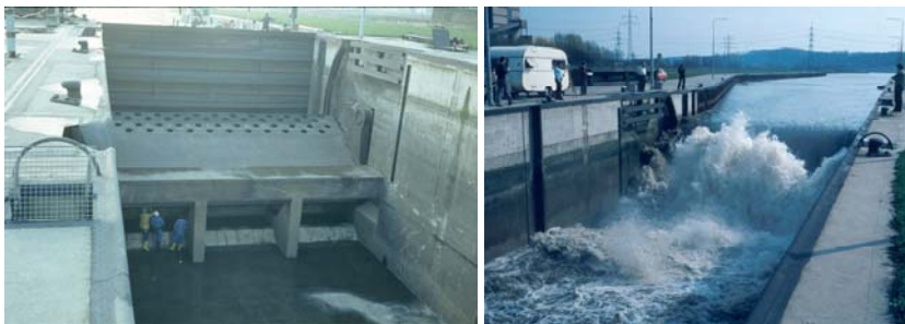
Fig. 16 - Upper gate at lock Lisdorf (D) during inspection and during a test for flood discharge
