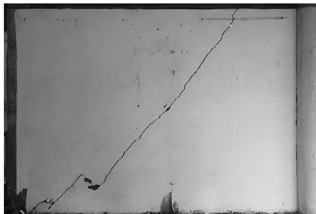
FIGURE 1 Diagonal shear cracks of RC walls in actual buildings after earthquake events. 1
