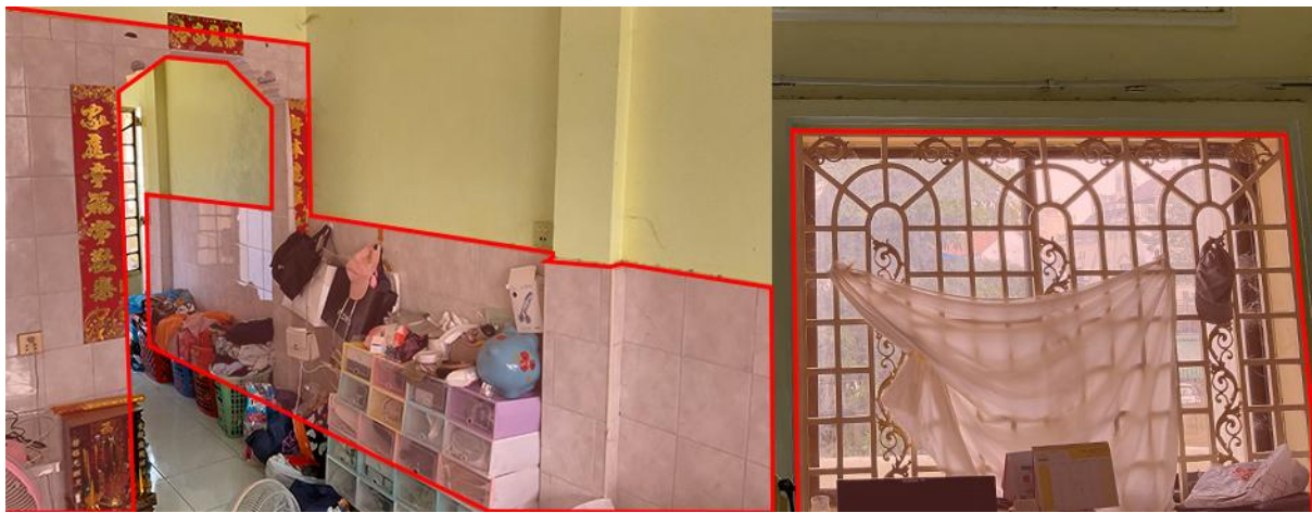
Figure 5-8. Ceramic tiles to be removed from the interior of the external wall (left) and steel to be removed from windows and doors (right).
