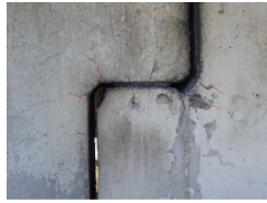
(b) Re-entrant corner crack (photo courtesy by SPW)
