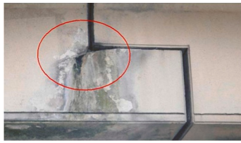
a) Connection in a bridge deck with a re-entrant corner crack and related deterioration (photo courtesy by SPW)
