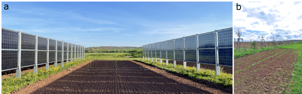
Fig. 5 Vertical AgriPVplus demonstrator in Wallhausen, Germany: (a) strip cultivated with spring wheat in the AV facility and (b) spring wheat in the reference zone
