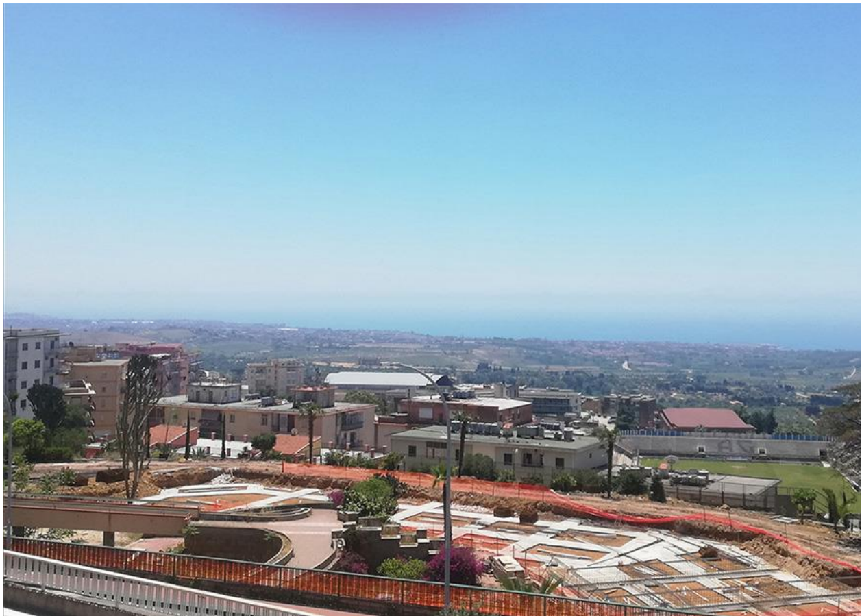
Figure 7. Panoramic view of the area. In photo the excavations work and new concreting are clearly visible (photo by T. Cilona - May 12, 2024).
