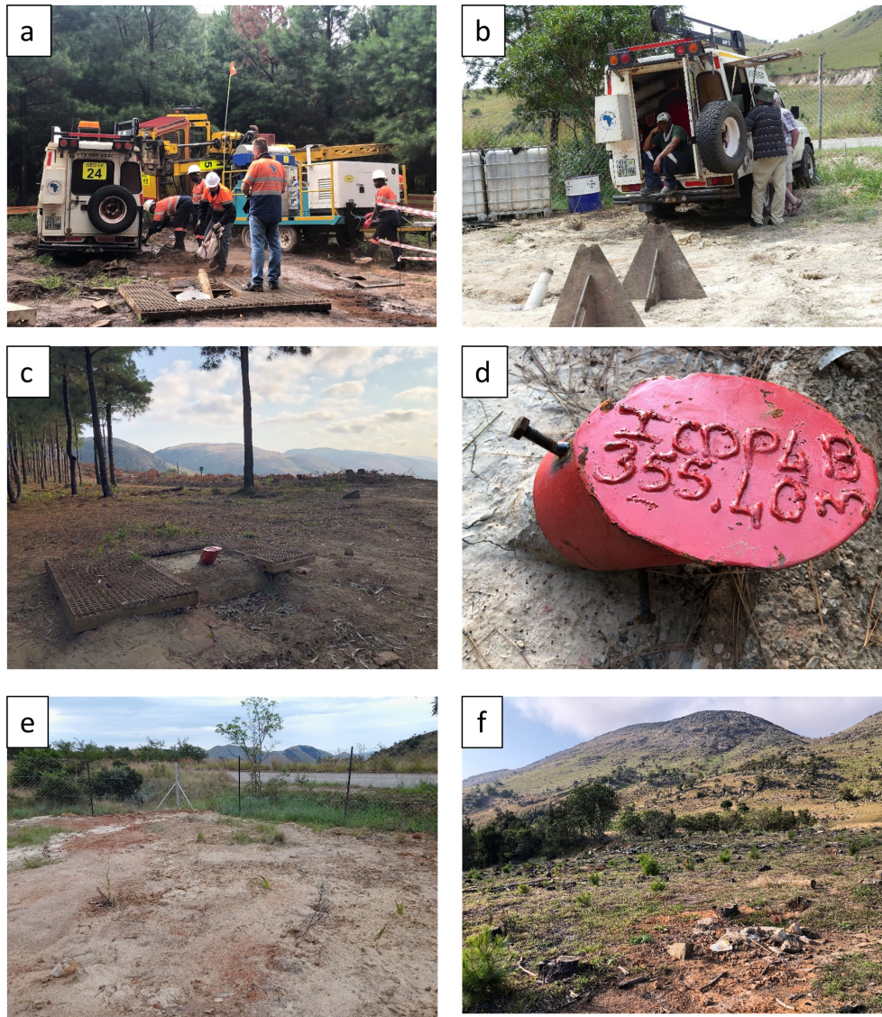
Figure 9. Post-drilling site operations. (a, b) Logging. (c, d) Site 4B with the cap welded on; the steel grating is yet to be removed. (e) Site 2 with the equipment removed; the site still needs to be raked and the fence removed. (f) Site 4C rehabilitated.
