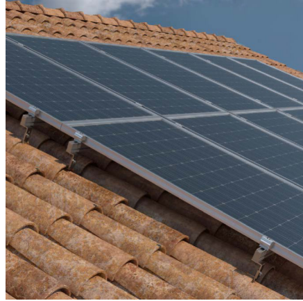
Figure 7: Alternative solution: solar panels overlapping the existing roof, allowing the integrity of the roof and its traditional materials to be preserved with a very modest elevation of the whole.
