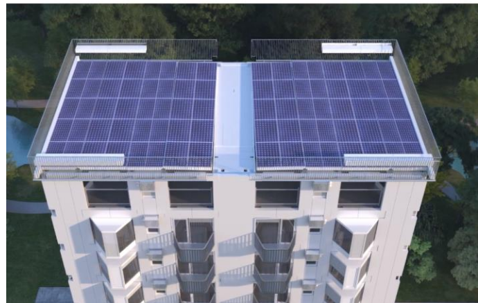
Fig.6 ROOFTOP PV SYSTEM
