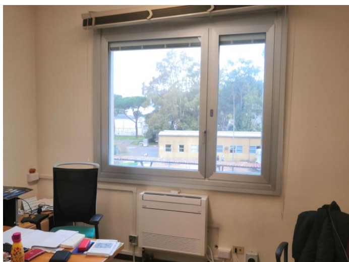
Fig.4 VIEW OF A TESTING ROOM, THE DYNAMIC WINDOW AND THE INTERNAL UNIT OF THE EC SPLIT SYSTEM
