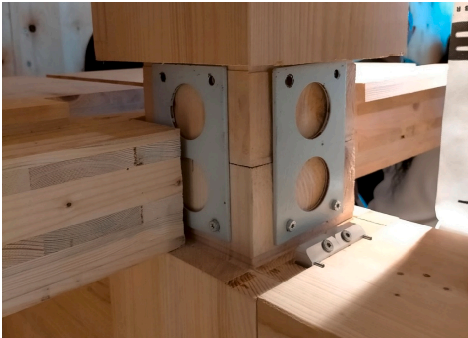
Fig. 1. Example of a bolted beam-column and slab-column connection that allows disassembling and reassembling.
