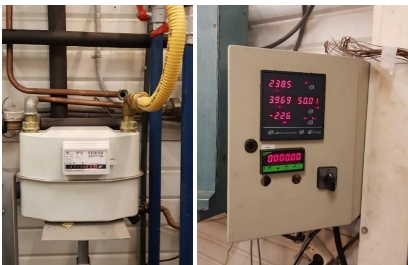
Figure 41. Gas and electrical metering installations on the test bench.
