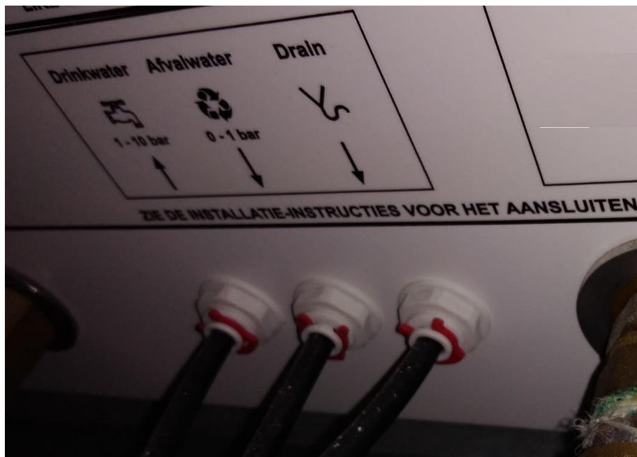
Figure 32. Photograph of the back of the system, with the two water excess evacuation pipes (and the water supply pipe).
