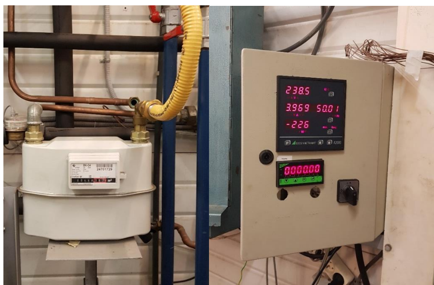
Figure 78. Gas and electrical installations.
