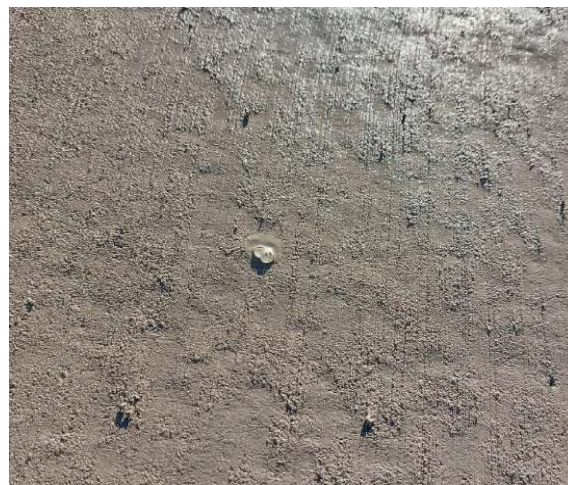
Figure 4 - Bleeding craters appearing on the concrete surface, mostly when high placement speeds are used
