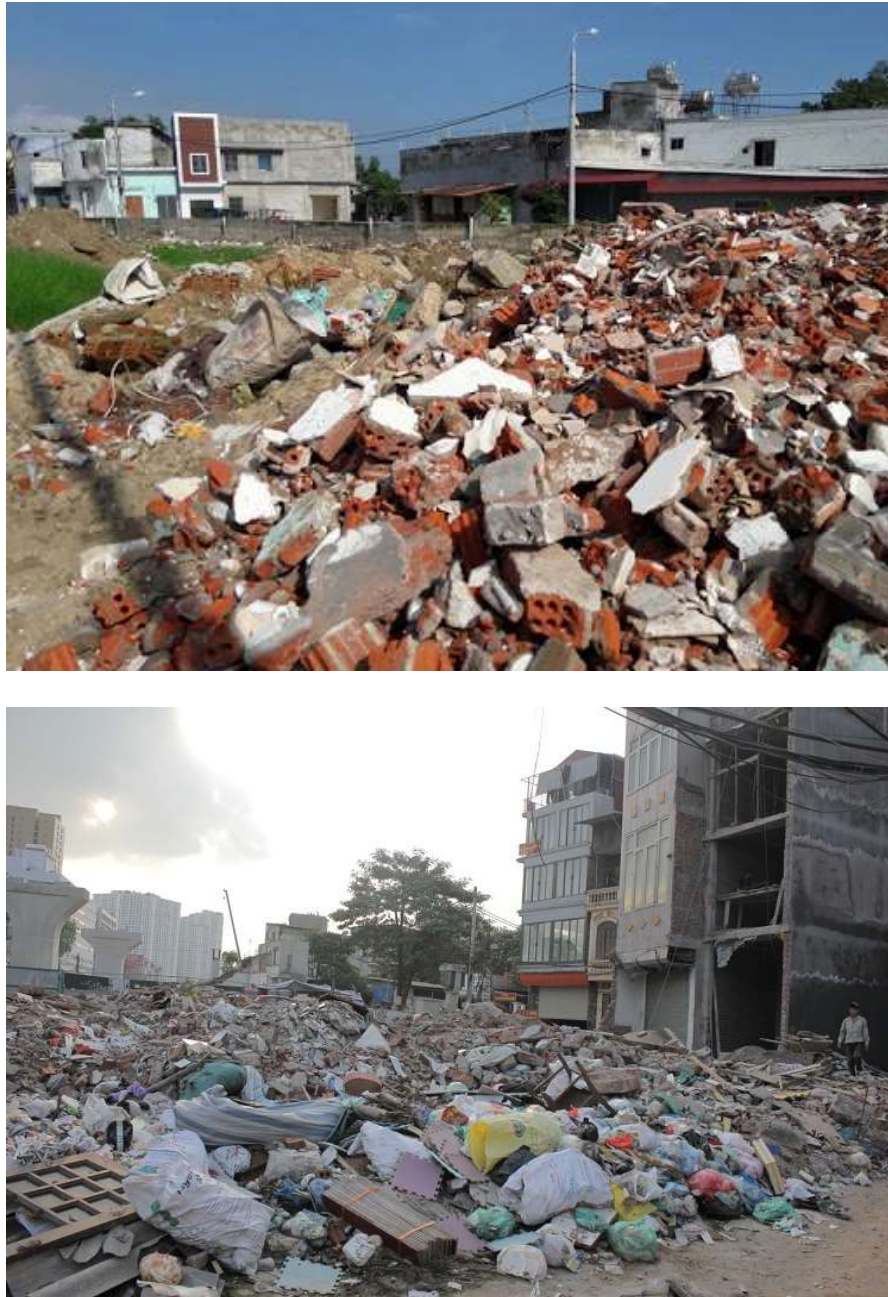
Figure 7: Construction waste and its dumping on the street cause unsightly environmental damage.
