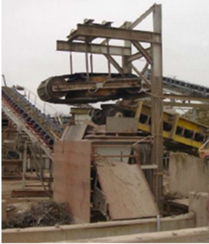
Figure 7 : electromagnet band for extracting steel
