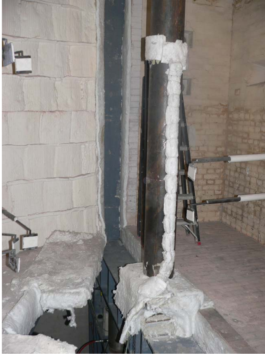
Figure V-11. Fire protection of the strain gauges of the test FRFC 3A
