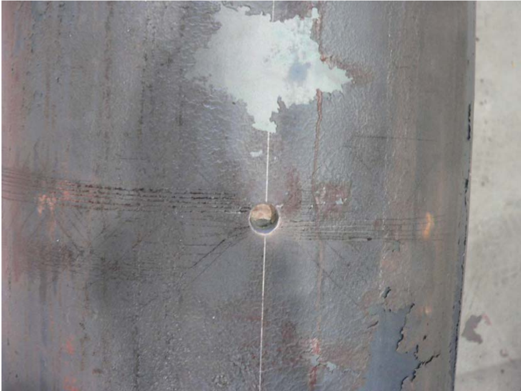
Picture A2.11. The movement of the mark in concrete at the steam vent.
