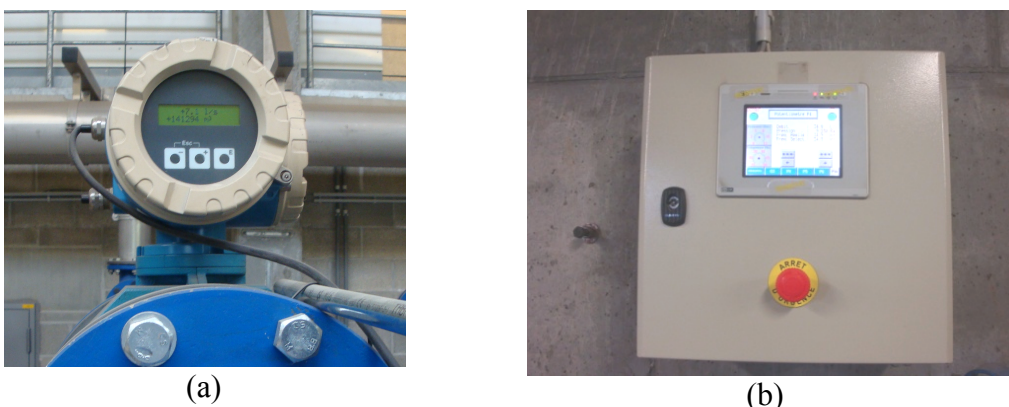
Figure 3.9: Photos of the flowmeter (a) and the control panel of the pump (b)
