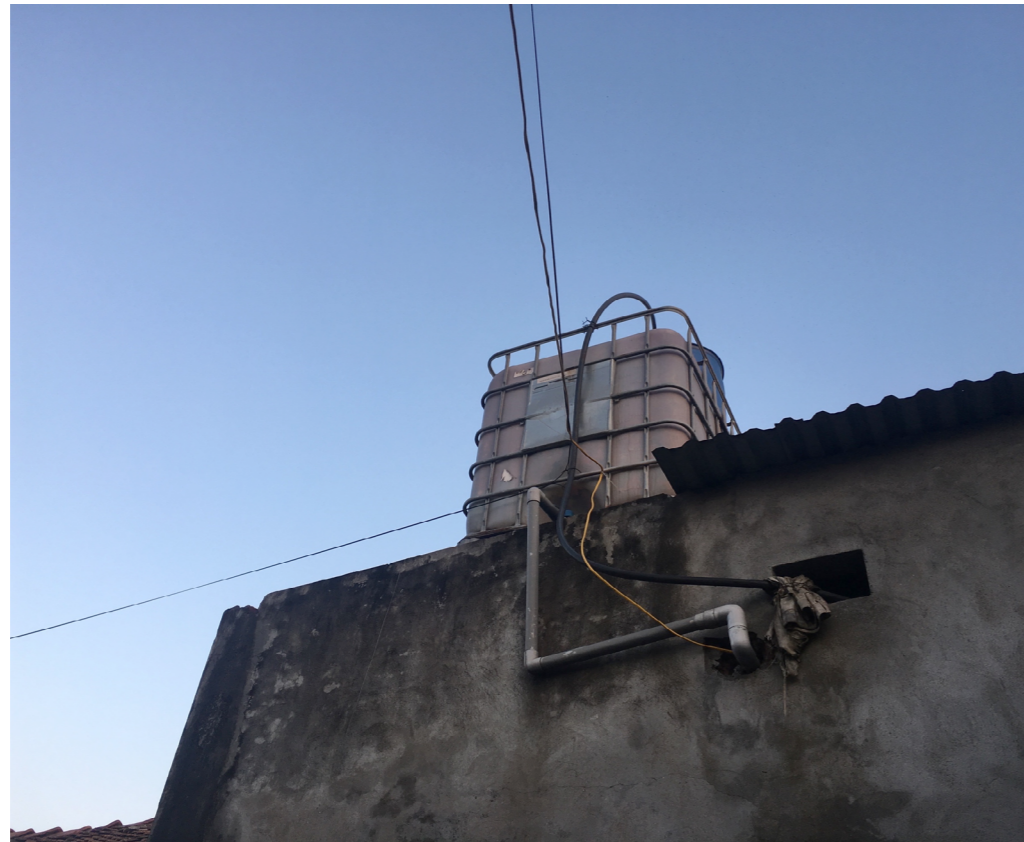
169. Hanoi. Water storage tank on the rooftop.
