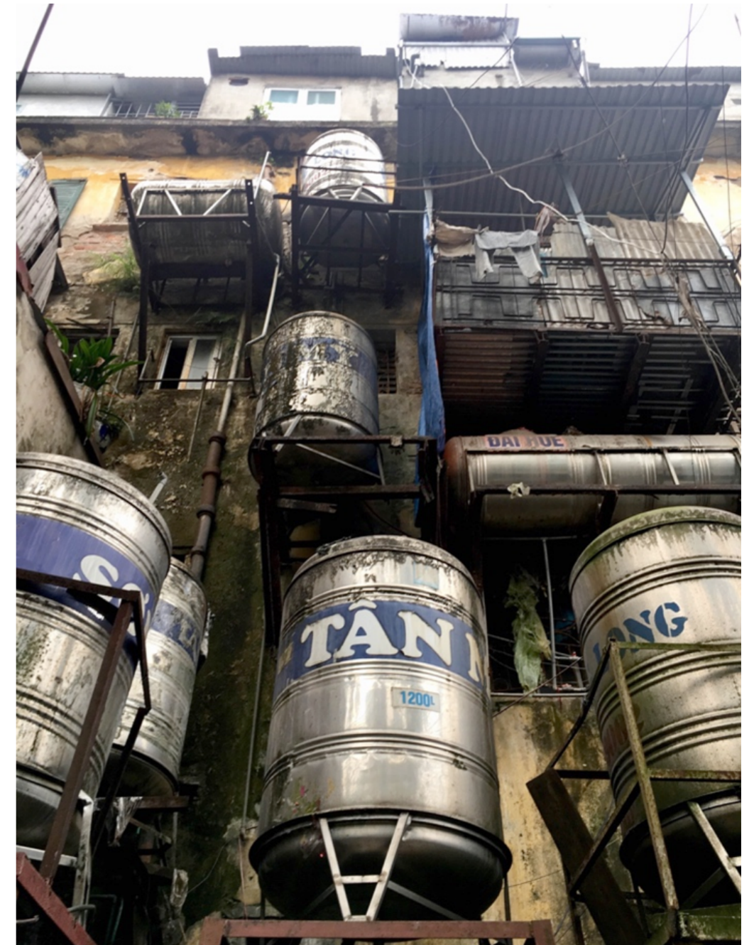
111. Individual water tanks installed in NCT north building facades
