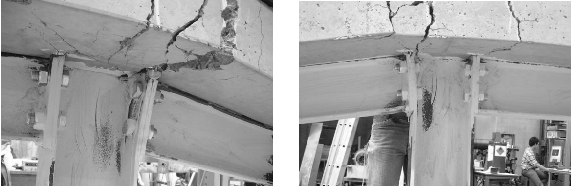
Figure 29. Spread of yielding in the steel components of the external composite joints
