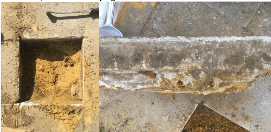
First excavation (Watermael-Boitsfort, Bruxelles) - Left: Removal of the concrete slab. Right: Concrete slab and profile mortar thickness. Images by Sylvie Smets
