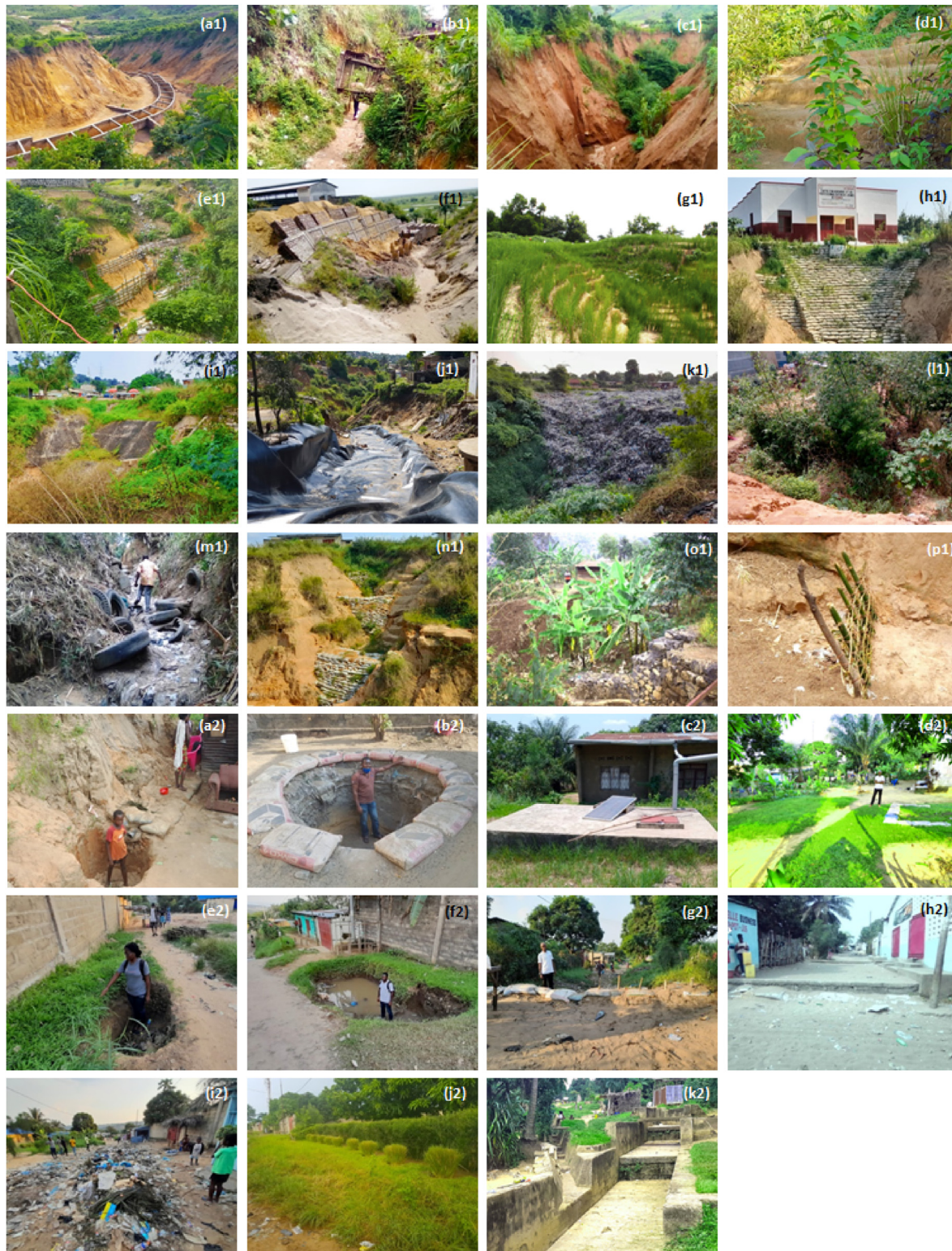
Fig. 4. Illustrations of measures taken to stabilize large urban gullies in D.R. Congo. a1: gully channel canalised with concrete; b1: vehicle wrecks placed in the gully channel; c1: planted vegetation in gully channel; d1 & e1: terraced gully walls; f1: supporting walls; g1: vegetation (vetiver) planted on gully walls; h1: sand bags to reinforce the gully head; i1: concrete spillway at the gully head; j1: plastic (geomembrane) or metal sheets to reinforce the gully head and start of the channel; k1: dumping household waste in and at the gully head; l1: vegetation (e.g. grasses, shrubs, crops) planted at the gully head; m1: small dikes of car tires in the gully channel; n1: sandbags placed in the gully channel (often in small piles); o1: gabion check dams in the gully channel; p1: diverse small sediment trapping structures in the gully (e.g. fences); a2 & b2: runoff retention and infiltration pits at parcels; c2: rainwater storage tank (also used for local consumption); d2: vegetation at parcels; e2 small infiltration pits along roads; f2: large water retention basin on a road; g2: small sandbag dams along a road; h2: small (stone) dams along the roads; i2: piled-up household waste along the road; j2: grasses and shrubs planted along the road; k2: runoff deviation channels in the upstream area.
