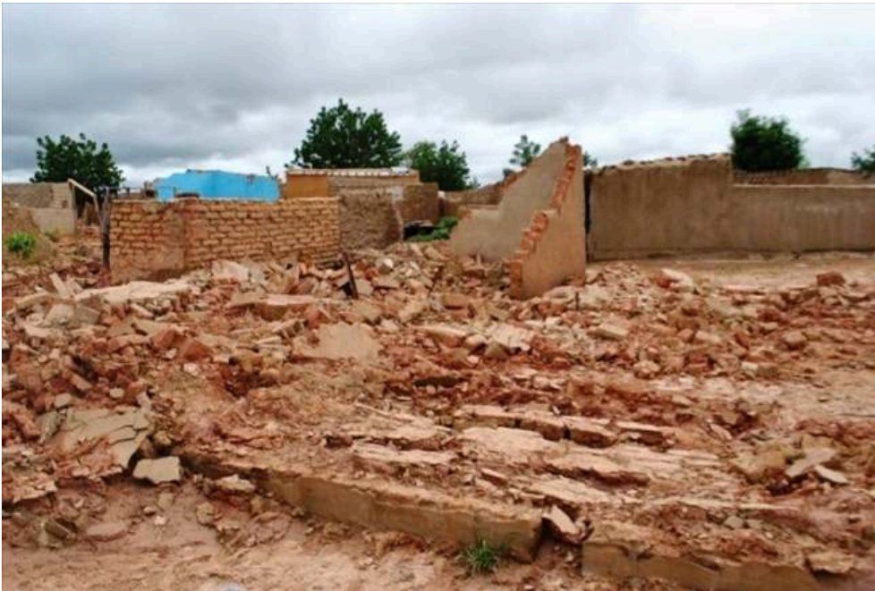
Picture 2: Collapsed house in the undeveloped area of Ouagadougou during the 2015 floods
