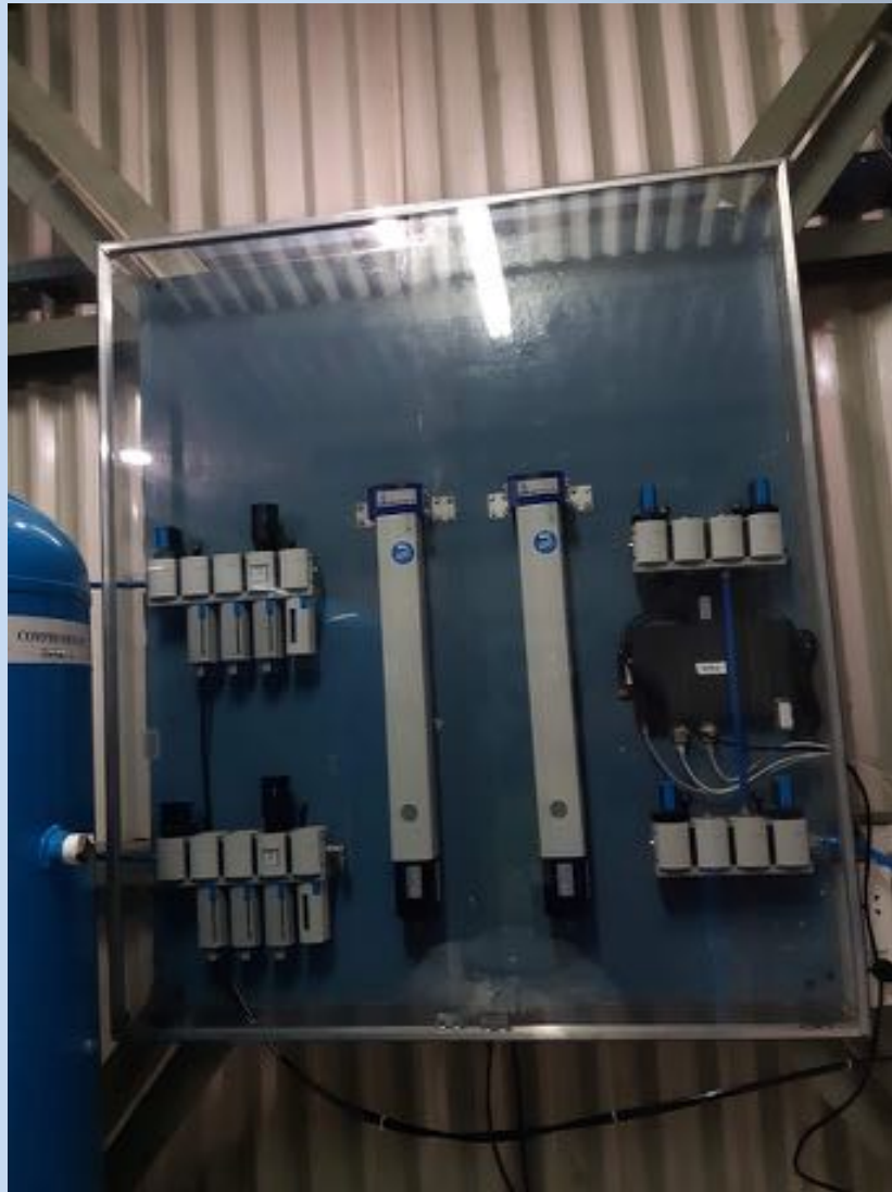
Pneumatic modules located near the 2 air compressors
