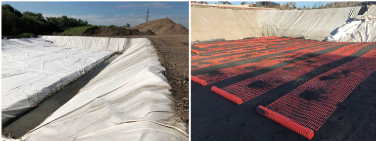
Figure 15. Pool for sludge drying (left) and its sand bed (right)
