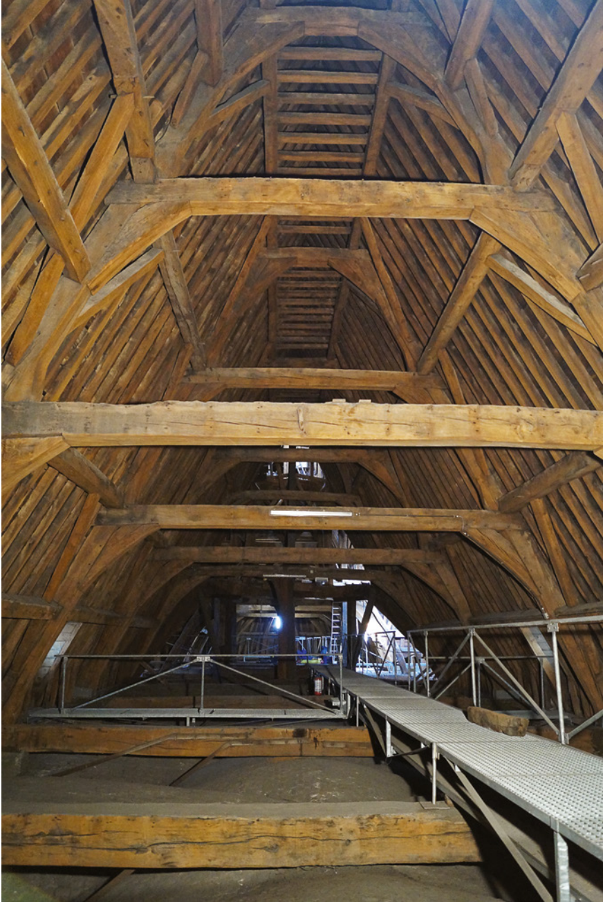
FIGURE 8 General view of the framework of the nave of the church of Notre-Dame du Sablon
