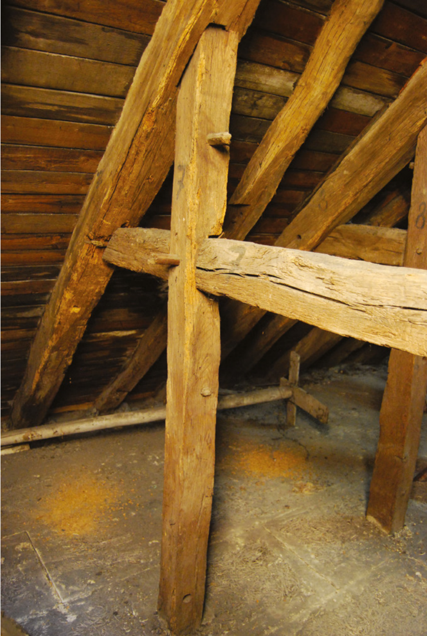
FIGURE 6 Frame covering the nave of the church of Saint-Lambert in Woluwe-Saint-lambert © S. CREMER, WORKING PHOTO, KIK-IRPA, URBAN.BRUSSELS
