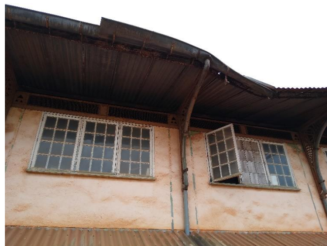
Figure 16 : view of some deteriorated roof edge purlins of the courthouse building of Mbanza-Ngungu.
