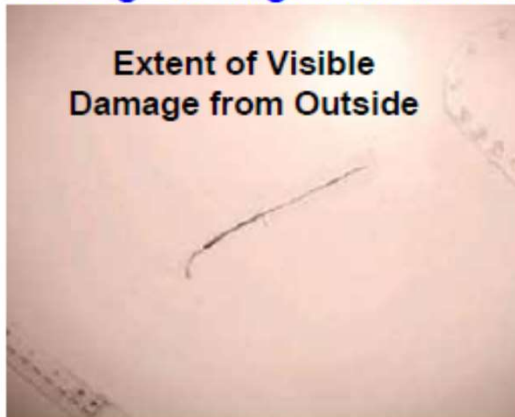
Damage from ground vehicle
