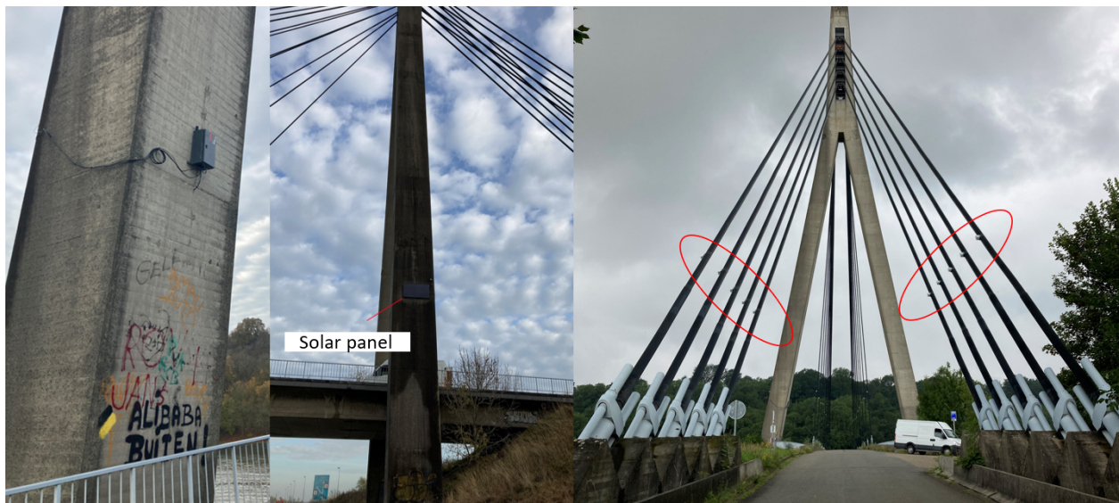
Figure 7: Photographs of the LYRA system attached to the Lanaye bridge showing the central station (right), the solar panel (center) and the wireless nodes attached to cables LG11 to LG15 and MA11 to MA15 (right)
