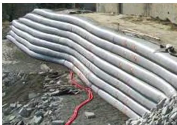
Figure 2.18. Construction phase of a retaining wall with a facing made of geosynthetic tubes filled with granular material [GOR 15]. For a color version of this figure, see www.iste.co.uk/grange/soil.zip
