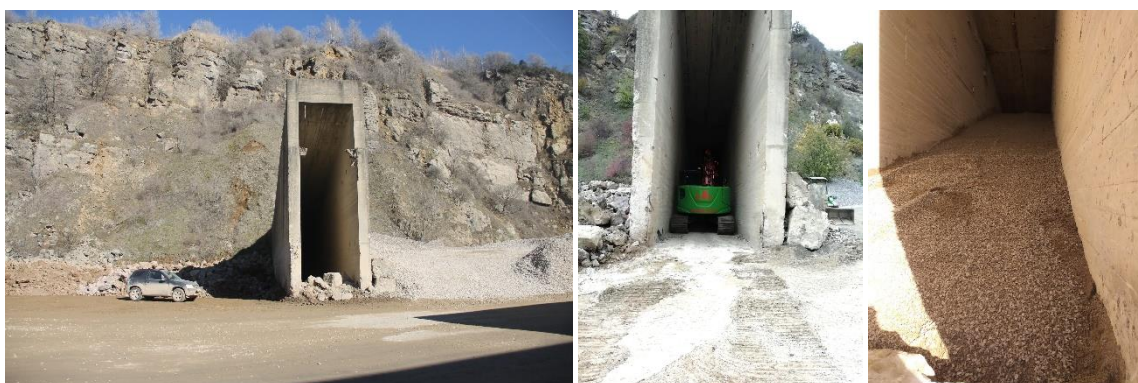
Figure 34. Old milling installation at Marche les Dames prior, during and after securisation.
