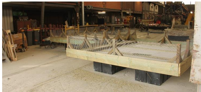
Figure 33. Finalised platform at Lessines prior to positioning on the quarry's old inundated pit.
