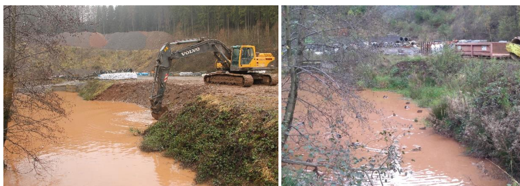
Figure 32. Sloping / creation of high waters in a technical basin at Warche quarry and its use by ducks in winter 2020.
