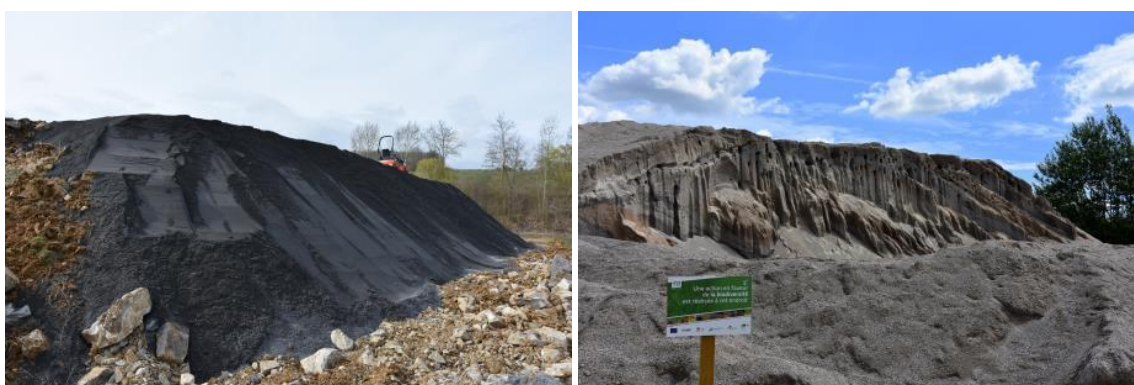
Figure 14. Vertical face under construction at Moha and functional vertical face at Les Petons.
