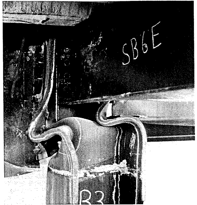
Fig. 8. Local buckling observed at Cardington (test by BRE).
