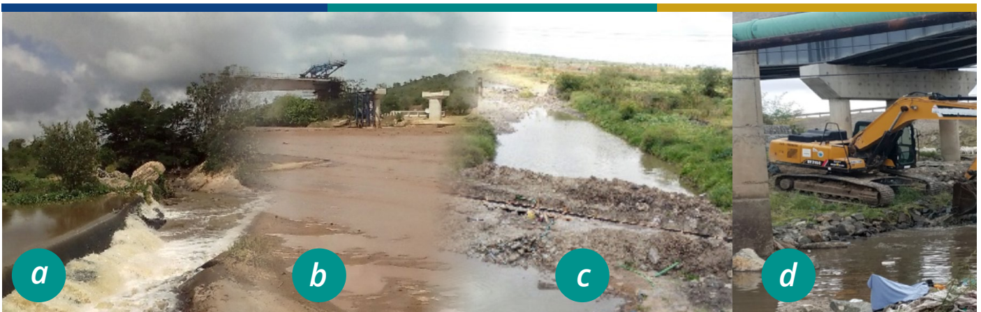
Figure 4: Habitat modification a) barrier bridge at Kiaone, b) Baricho bridge under construction, c) barrier and d) bridge construction at stony Athi, Athi River, Kenya
