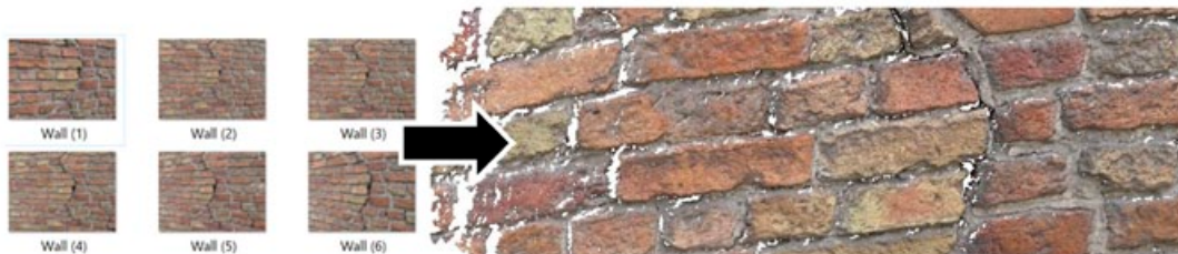
Figure 1. Point cloud generated from photographs of a wall with a MVP software.
