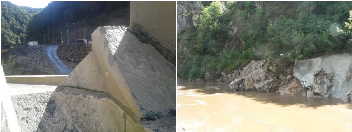
Figure 9: Flip bucket abrasion (left) and left river bank erosion (right) after bottom outlet operation at design discharge ( 265 \text{ m}^3/\text{s} )
