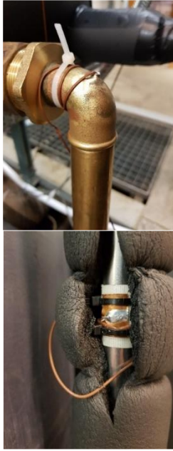
Figure 4: Thermocouples immersion sleeves: surface and elbow thermocouples
