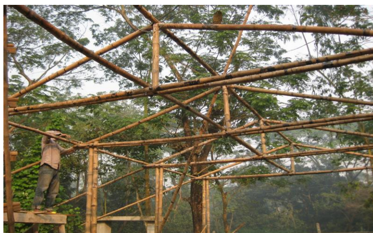
Figure 7. Photo of a bamboo treatment and building workshop with the Rajapur community.
