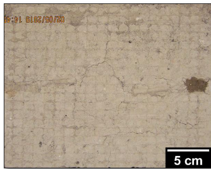
b)-Cracks appearance at the bottom of the sample
