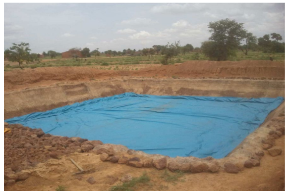
d) Pond with covered bottom and waterproofed cement walls in Yatenga province
