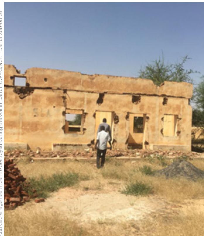
Abu Gao village health centre destroyed during the war in Darfur. ©WHO/North Darfur Sub-office
