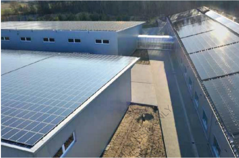
All roofs on the 4120m 2 of this warehouse complex, built by Mattig & Lindner in Germany, are entirely covered by photovoltaic solar panels.
