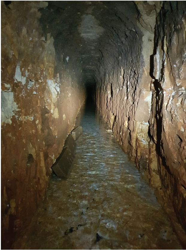
Figure 4. One of the “lateral” galleries in the Cretaceous chalk of Hesbaye still in use for the water supply of the City of Liège by the Public Water Company of the Liège area (“Compagnie Intercommunale des Eaux de Liège” CILE). Photo by Serge Brouyère.
