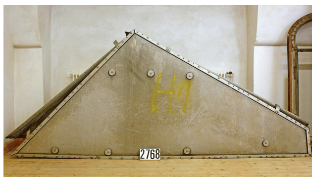
Fig. 1: Historical roof element of the Olympic Sports Facilities in Munich from 1972, Plexiglas® GS 215 stretch-formed, aluminum frame and round buffers that connected the sheet to a net of steel wire. Due to degradation, the once transparent, stretch-formed material became opaque and soiled.
