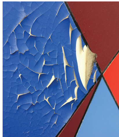
Detail of flaking paint of the integration Kalota. ©TROY-BRIGANTI.
