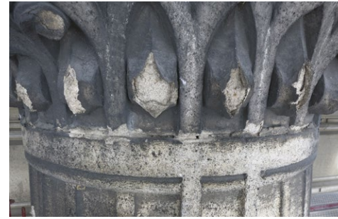
Capital, Deterioration of the Euville limestone, 2013*.
