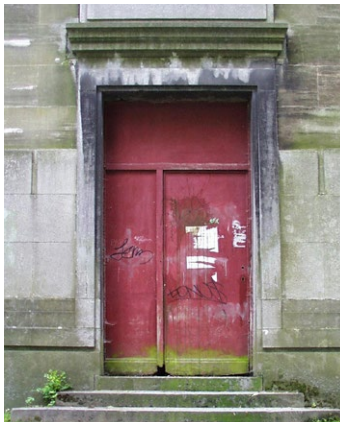
Exterior view of the rear door, before restoration, 2003*.
