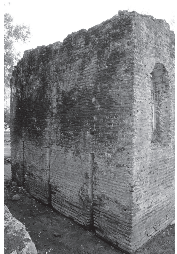
55. View of the rear of the apse, with grooves and piercing for the water inlet.
