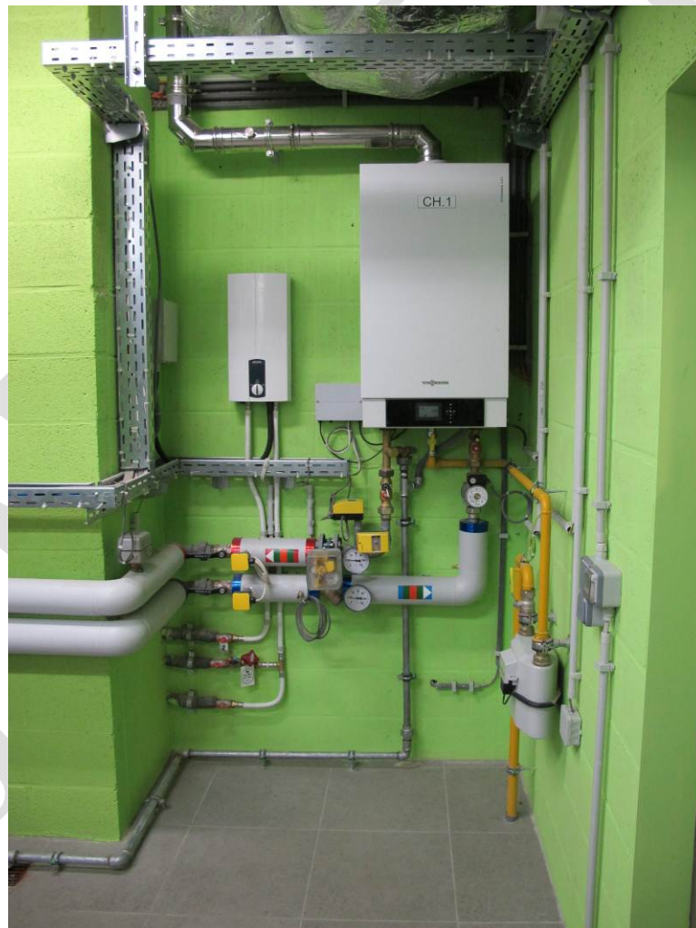
Figure 4: Heat production by a condensing boiler (right) for heating, and an electric water heater (left) for hot water
